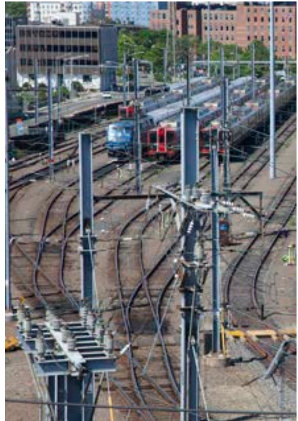
Electric Infrastructure in Stamford, CT
